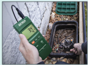
Measuring AC Magnetic Field output from sprinkler relay system
